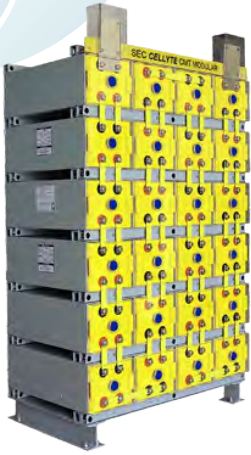
CELLYTE 2CMT/G Modular Steel Rack
